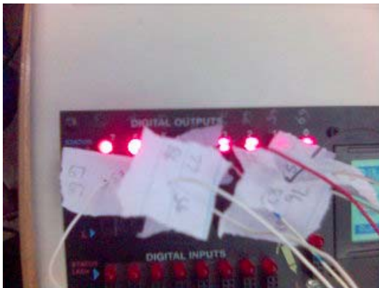
Inputs from switches
